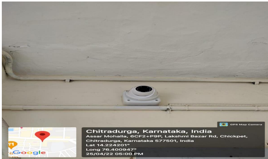
Figure 2 CCTV in front of Principal Office
